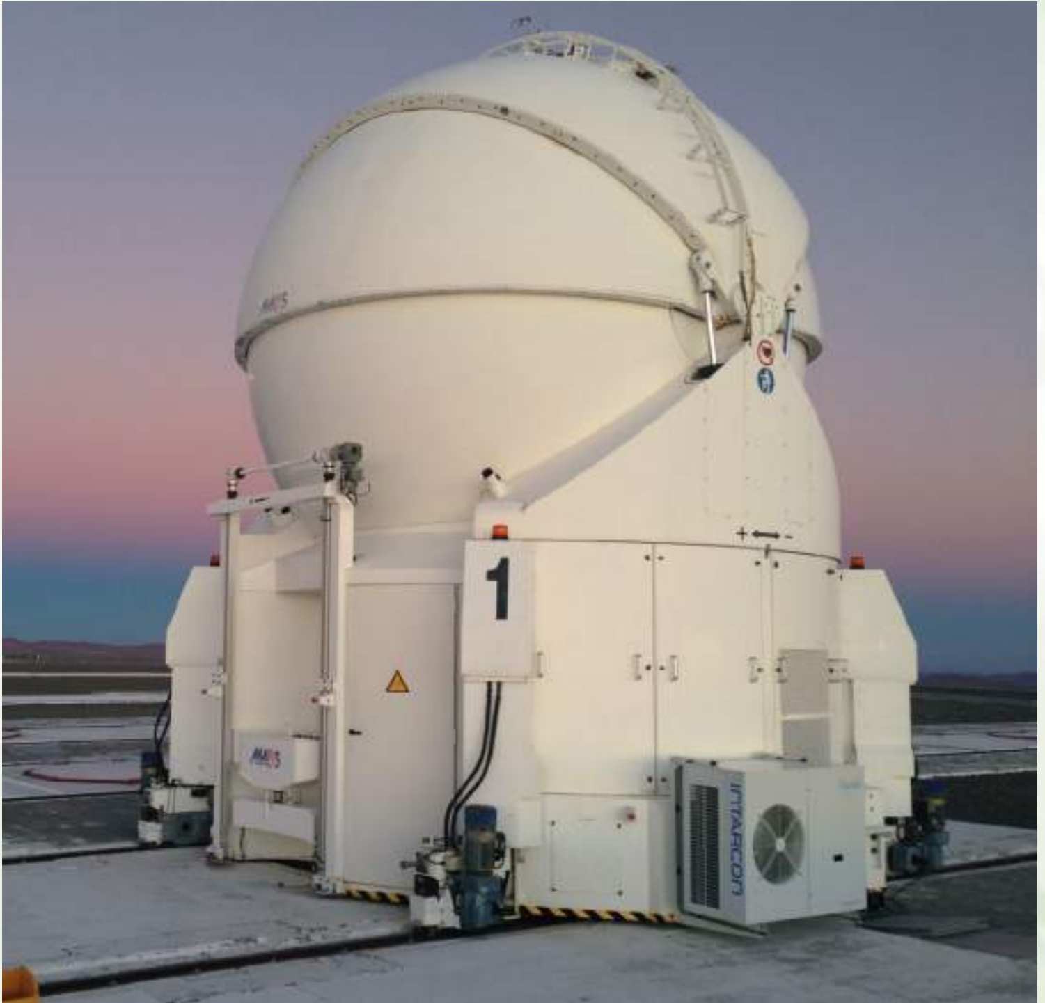
[ESO] Glycol chillers for Auxiliary Telescopes at Paranal site (Chile), 2013-2014
