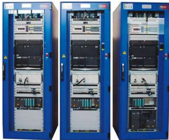
I&C Cabinets Procon Systems for ITER
