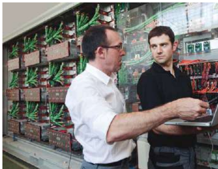
JEMA facilities ESS-Bilbao Project
