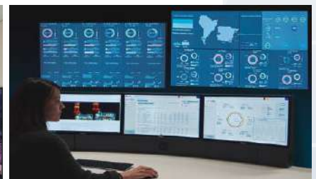
CMT Power Plants Monitoring Centre
