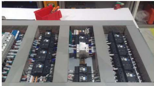
Lower part of the HSB01 distribution board
