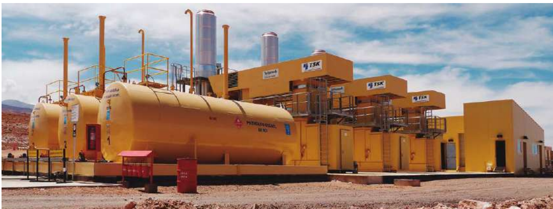
ALMA Multifuel Power Plant (2011)
