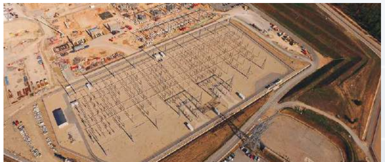
The very high voltage electrical substation on the south side of the platform (Photo IO EJJF Richie)
