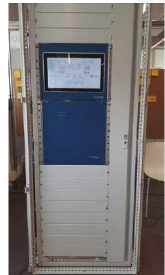
Cable Monitoring Interrogator
