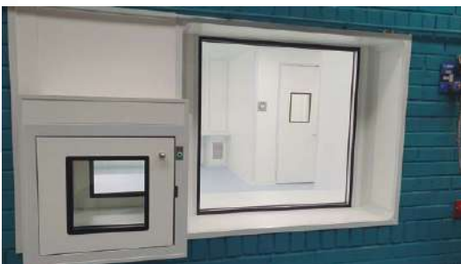
ARQUIMEA facilities - clean room
