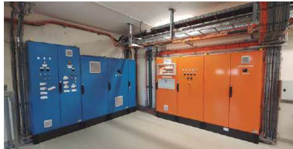
Electric cubicles - CERN AD TARGET
