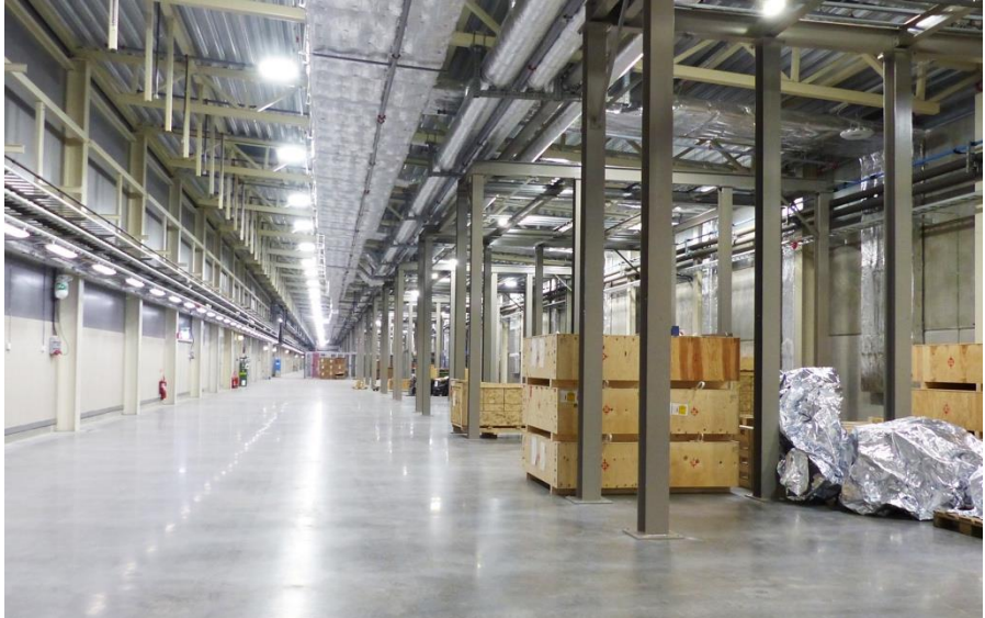
RF for normal conducting linac is installed, tested and in operation.
