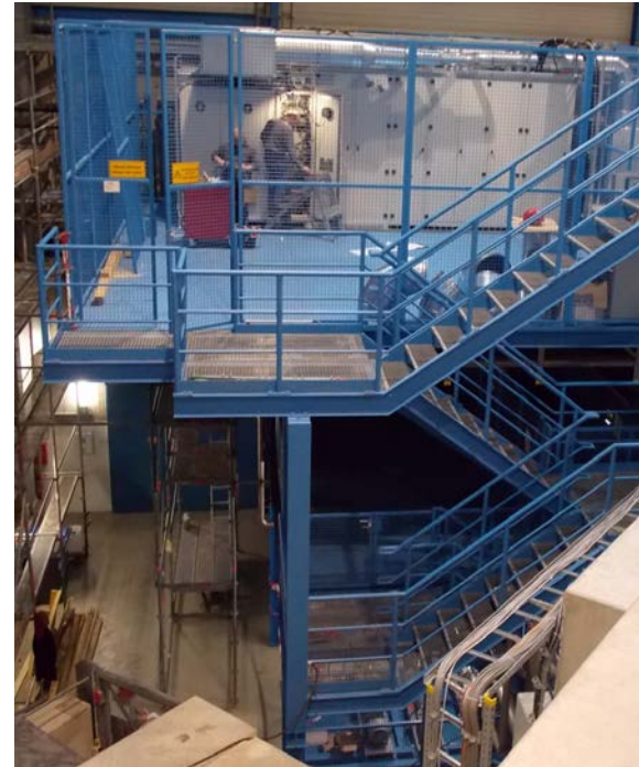
Platform for SIS18 h=2 power supplies (2 nd floor), mains distribution (1 st floor), and oil cooling system (ground floor)
