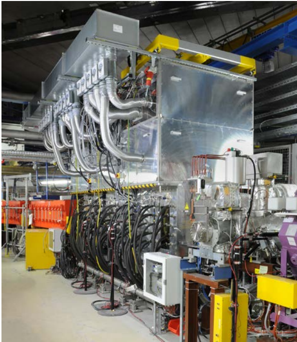
SIS18 h=2 cavities (tetrode power amplifiers on top)
