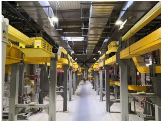
DC interconnection busbars
