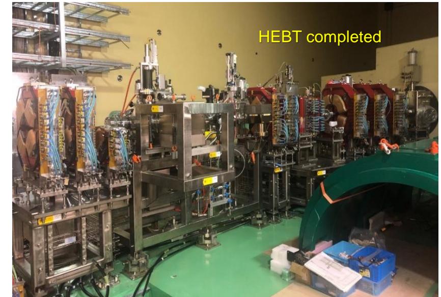
High Energy Beam Transport
