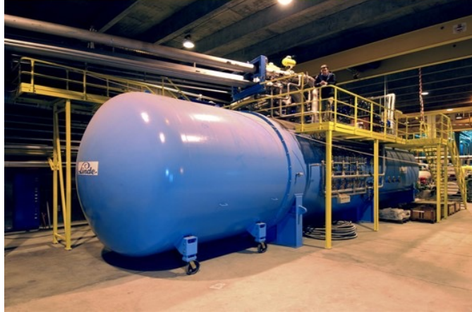
18 kW @ 4.5 K cold boxes (Air Liquide and Linde)
